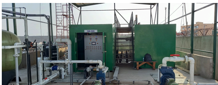
EFFLUENT TREATMENT PLANT WITH TERTIARY FILTRATION
