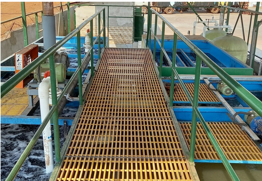
BIOLOGICAL TREATMENT STAGE, INDUSTRIAL EFFLUENT TREATMENT PLANT
