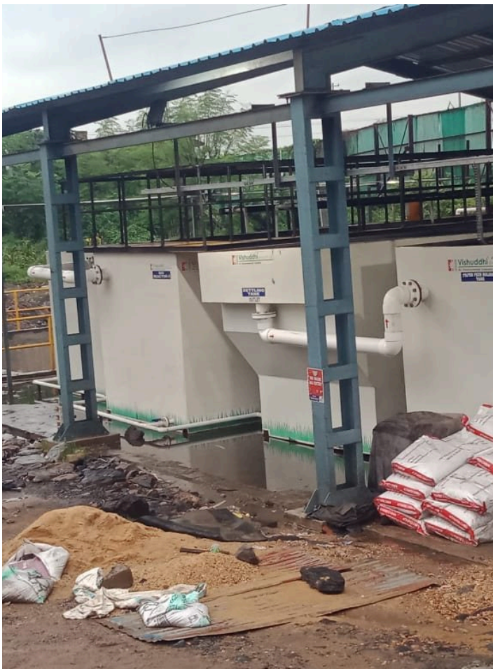
STRUCTURAL STEEL SHED AND PLATFORMS OVER PACKAGED PLANTS
