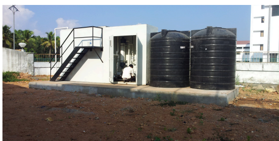
PACKAGED STP INSTALLATION
