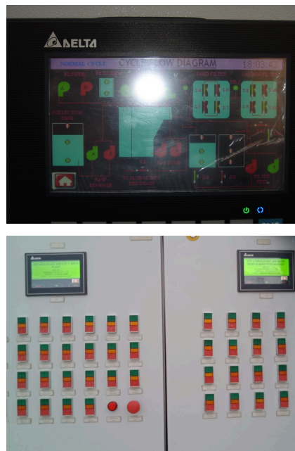
HMI SCREENS & PLC CONTROL PANELS
